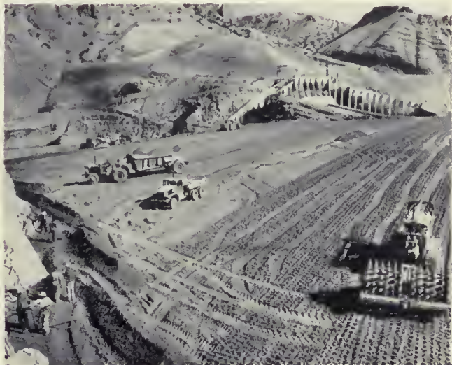
hauling equipment at right is stepping up the eventual water supply for 20,000 acres of land. Photos by T. R. Broderick.
